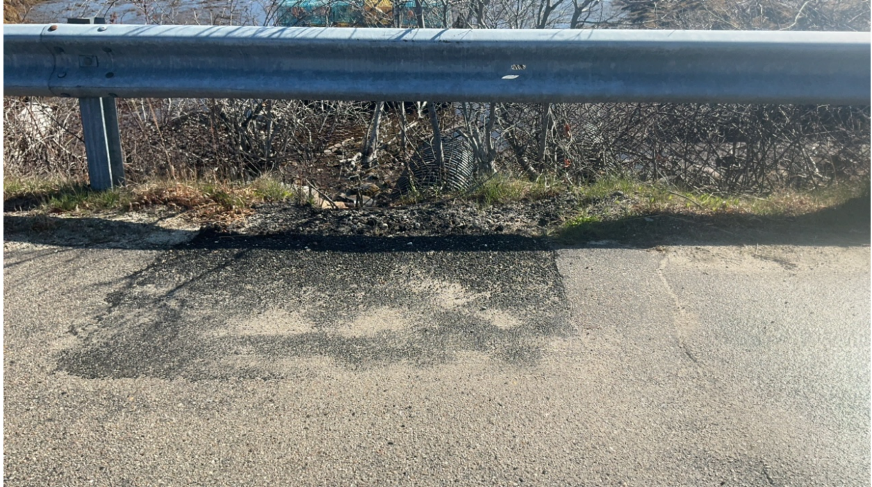
Figure 5: This section of Fern Ave above the culvert had to be patched after it was undermined and damaged during the 2024 winter storms.
