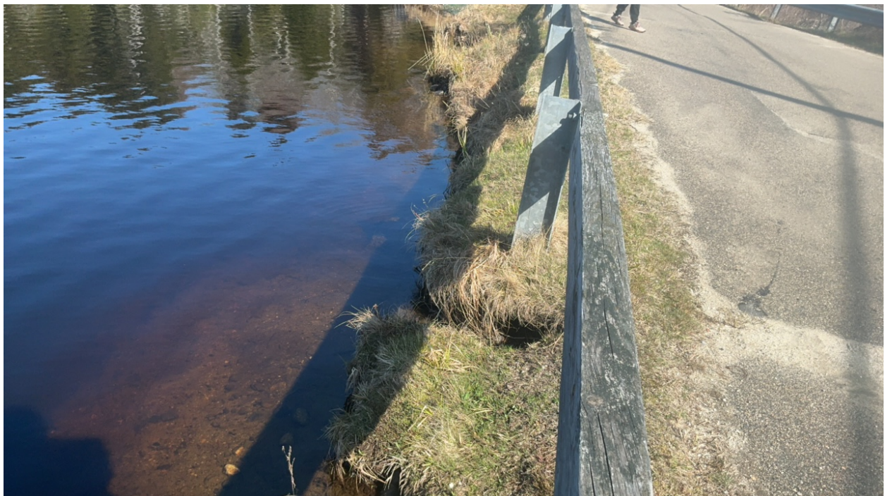
Figure 6: Runoff from the road has carved gullies into the pond shoreline.
