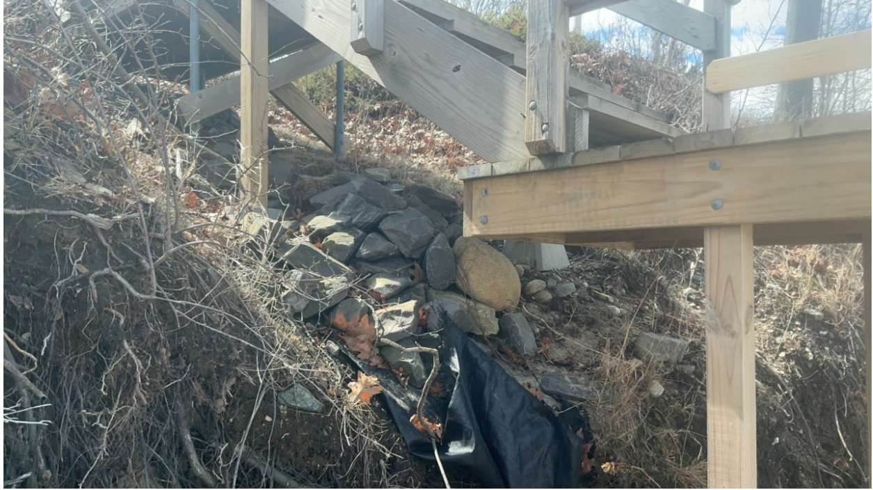
Figure 5: Gully beneath the shoreline access stairs and stone placed to prevent further erosion.
