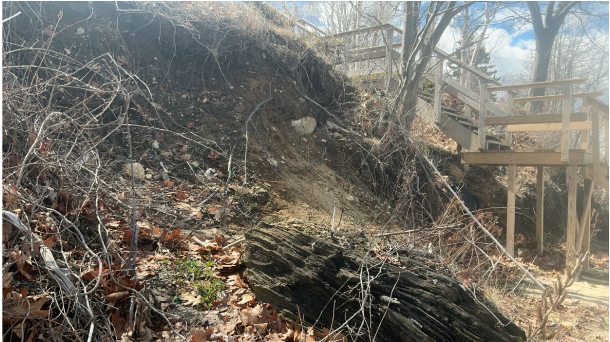
Figure 3: Bare soil and bluff erosion on the shoreline of the VFW Hall site.
