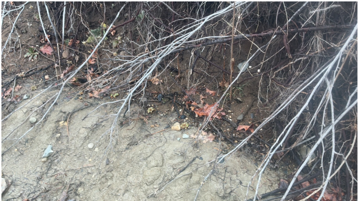
Figure 4: Photograph showing the two distinct soil layers of the coastal bank at the site. Small eroded channels called rills are visible in the bottom clay layer where groundwater is exiting the bank and running downslope.
