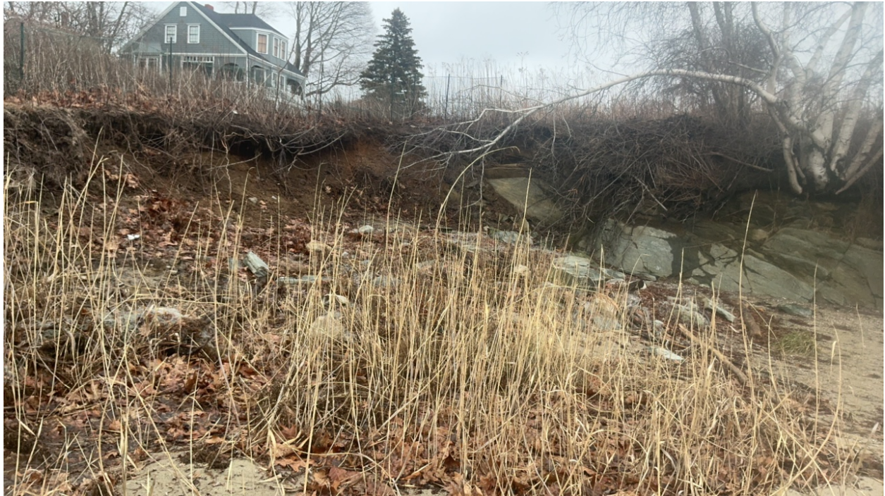
Figure 3: Southeast section of West Shore Beach where the sediment bluff meets bedrock.
