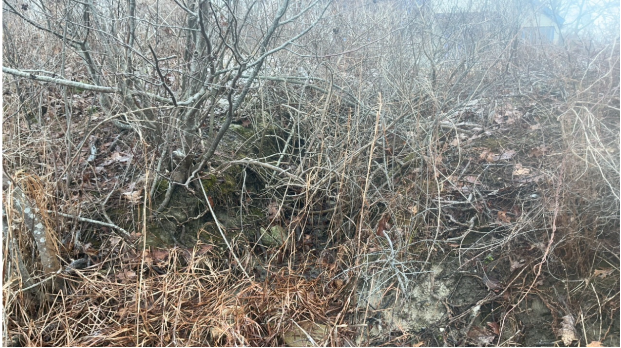
Figure 8: Photograph of a gully in the bank indicating surface water contributions to erosion.
