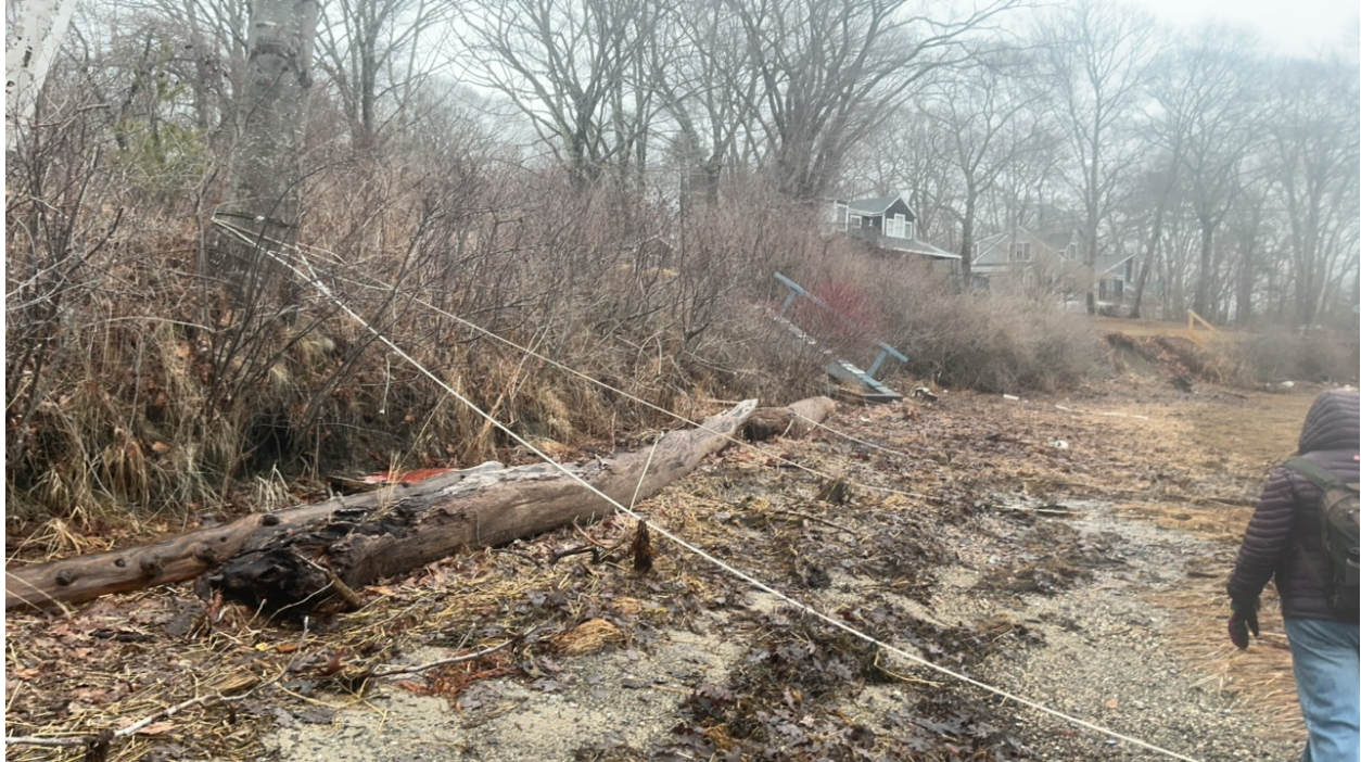
Figure 2: Photograph of the site shoreline facing north. Toe erosion including mild undercutting is visible on the bank.
