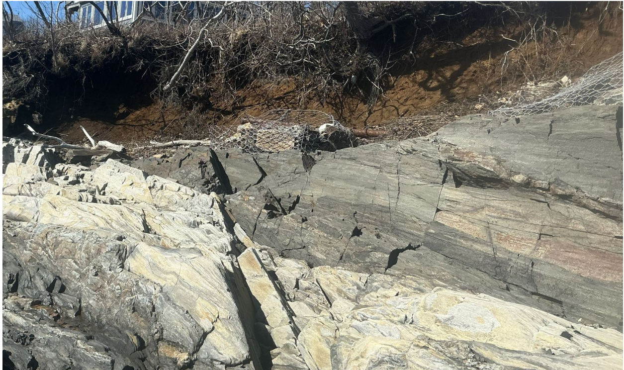
Figure 5: Erosion has formed a steep slope with bare soil on this section of shoreline.
