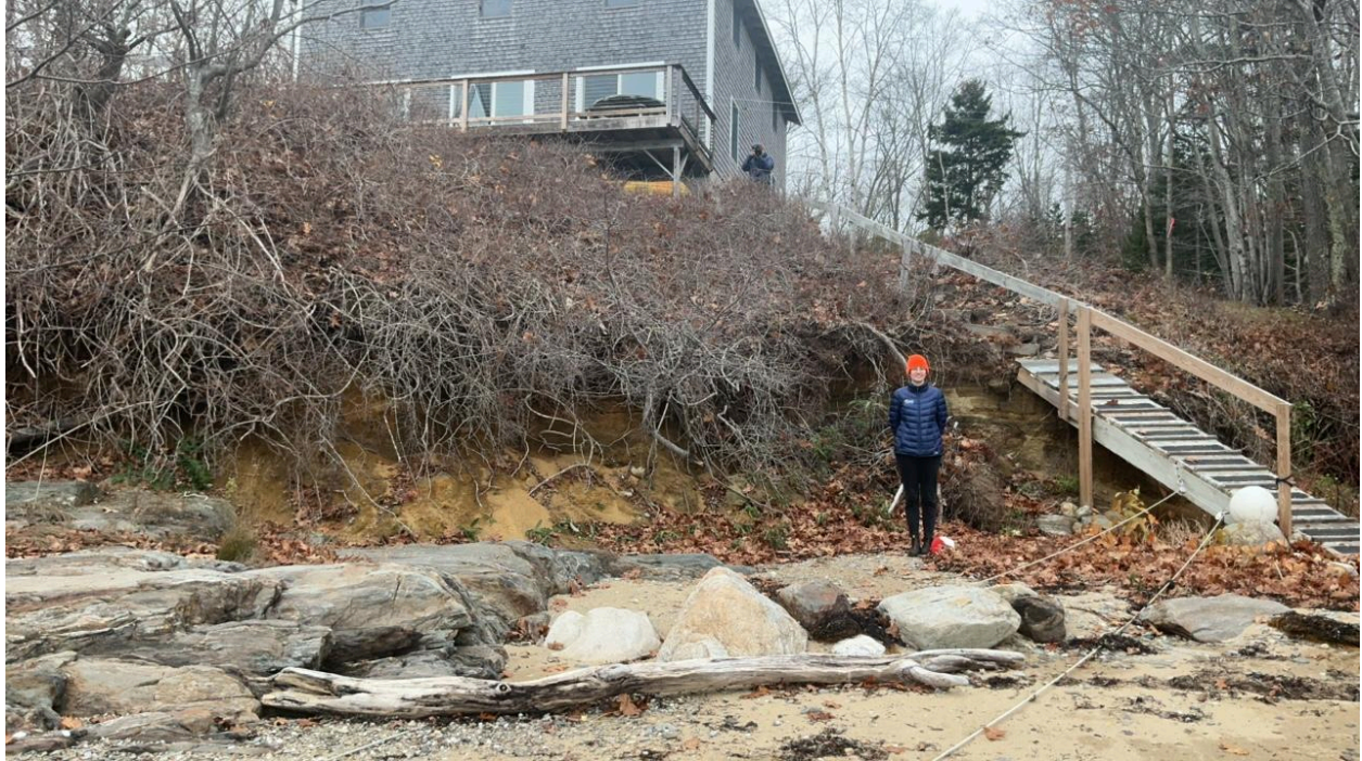
Figure 3: Partial view of the bluff and beach. Exposed soil and displaced soil blocks are visible.
