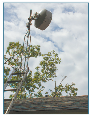
Microwave transmission tower, receiving internet transmission from Portland to Cliff Island
